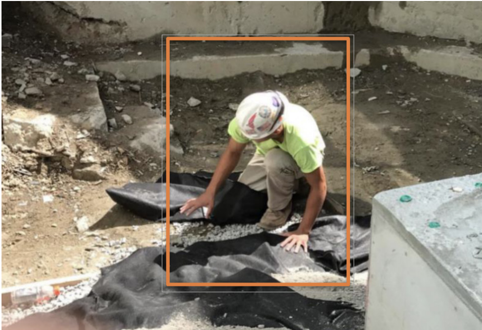
Suffolk has partnered with the startup Smartvid.io on technology that uses image recognition to detect safety risks like workers missing protective equipment. Courtesy of Suffolk and Smartvid.io
